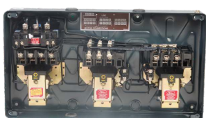
Interior View of MK1 SASD
