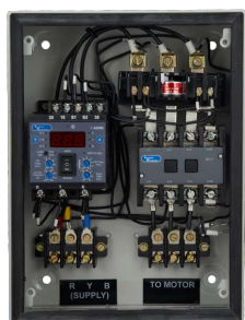
Interior View of MD Starter+ DOL Starter
